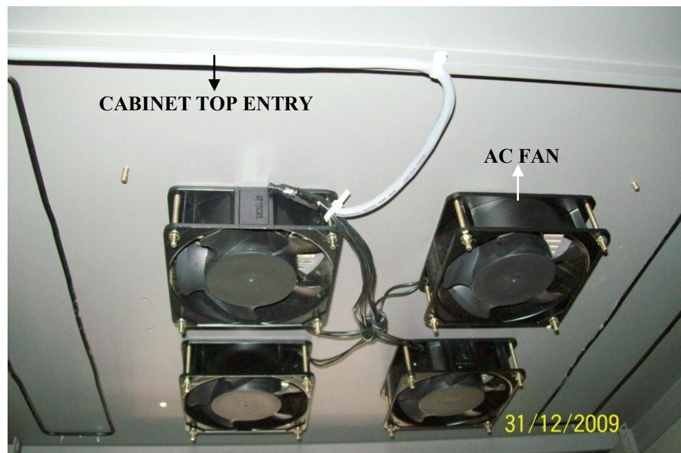
CABINET TOP VIEW
