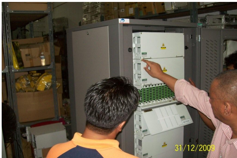
TM – HUAWEI – ONT CHECKING THE PANEL
