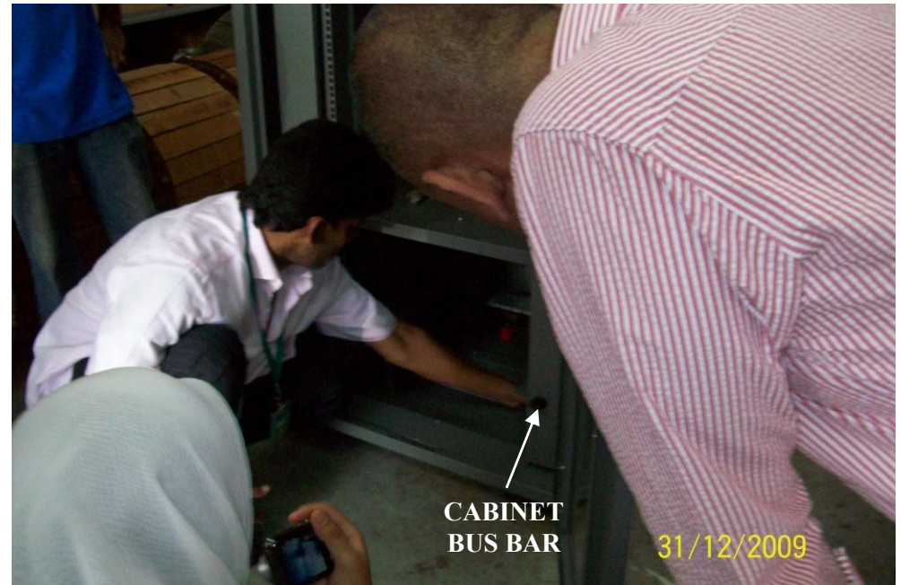
CHECKING CABINET BUS BAR
