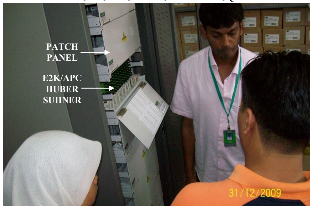
CHECKING METRO-E PANEL BOQ
