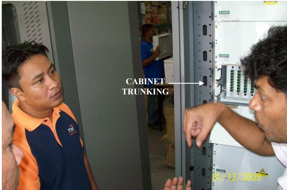
CABINET TRUNKING VIEW
